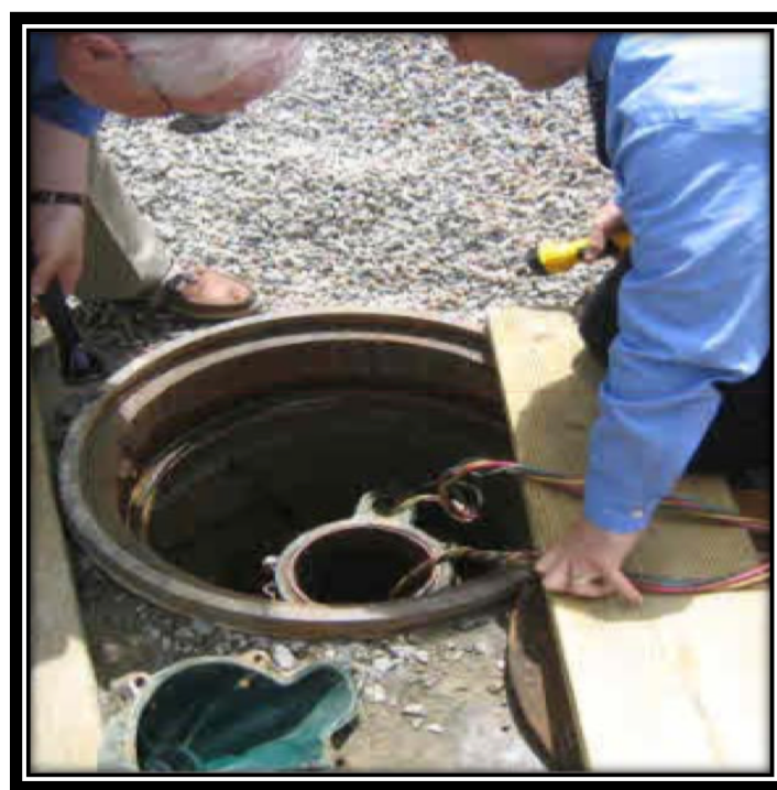
Figure 3: Geothermal wells at Harvard est. 2007 (Harvard)
